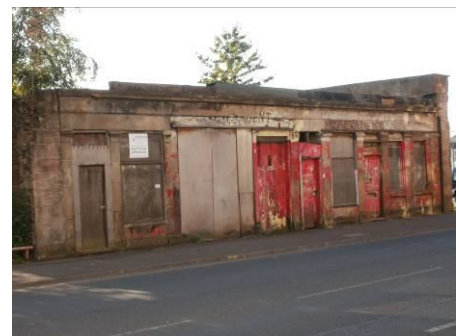
Derelict buildings on London Road
