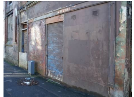
Derelict building on Stevenson Street
