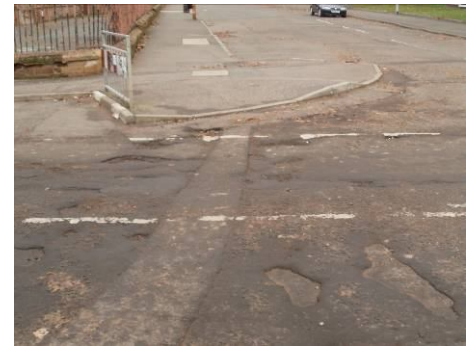
Poor surfacing on Green Street by junction with Stevenson Street
